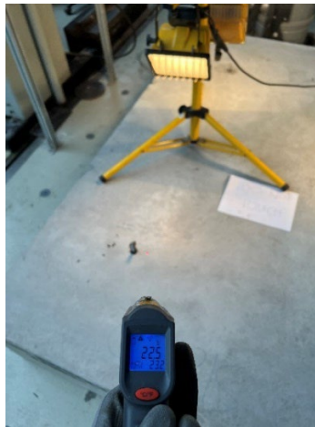
g) Heat lamps to maintain curing temperature Figure 2 Installation of anchor in concrete
