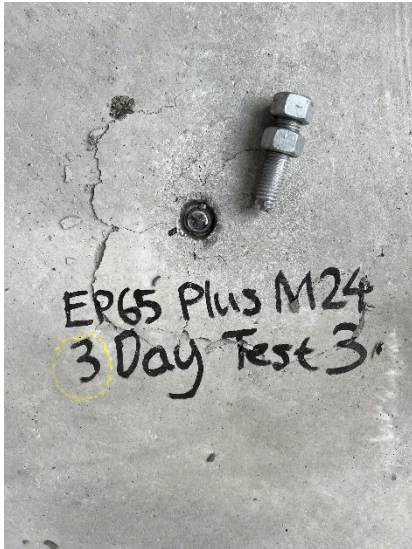
a) Steel failure
